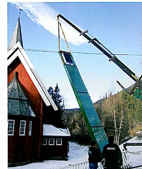
Solfangeren heises på plass utenfor kirken. Solar collector is erected outside the church.
