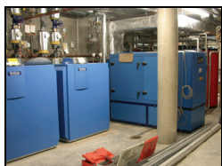
condensing boilers and CHP
