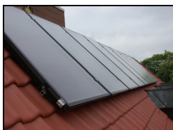
Thermal solar plant
